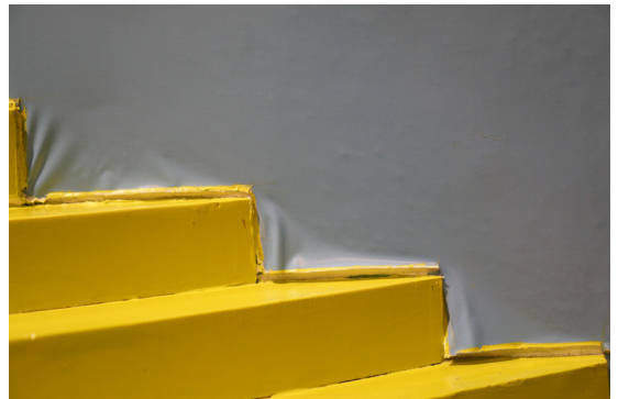
The exposed edges make it dangerous for children in the space
