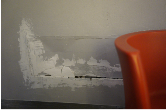
The damage to the walls can be dangerous and is also unsightly
